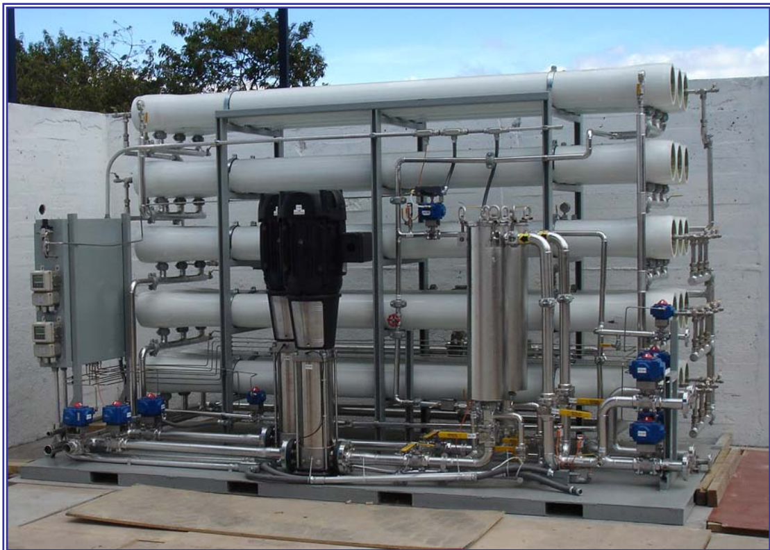
New Logic's S-18000 Spiral Membrane System Installed
