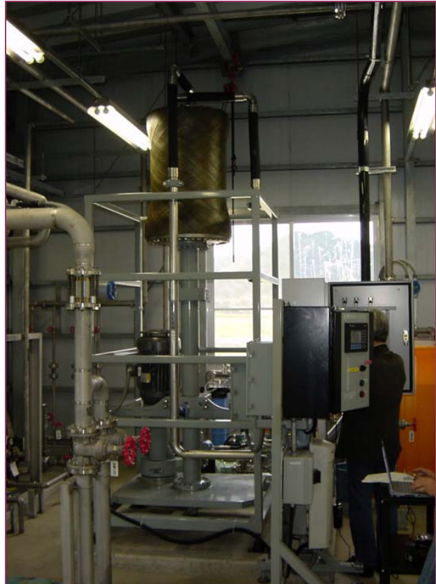
VSEP System installed for Manure Treatment in Japan
