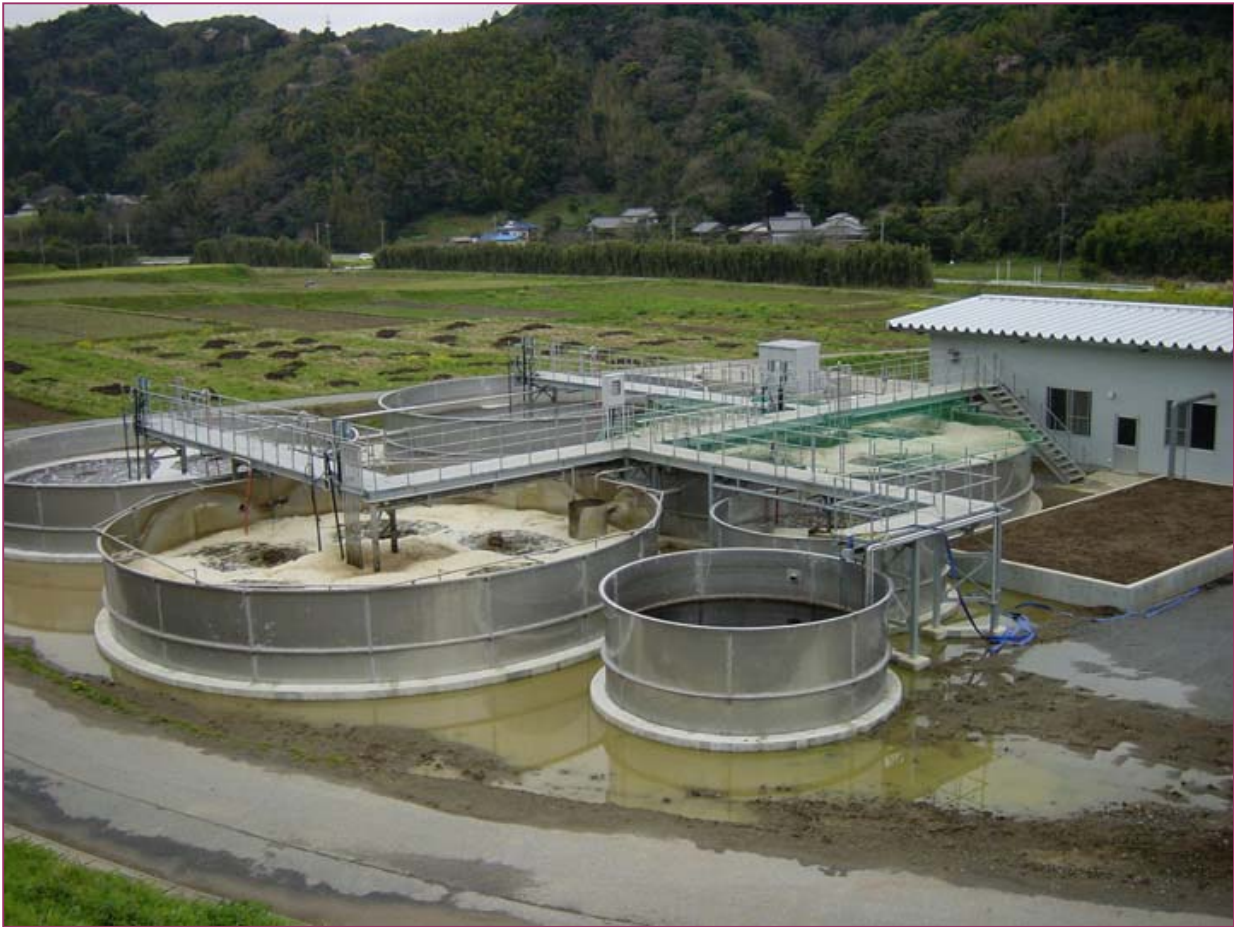
Typical Outdoor Aerobic Digester (Japan)
