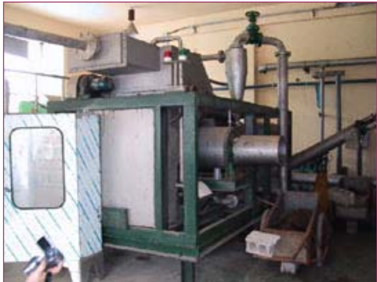
Typical Degritting Device
