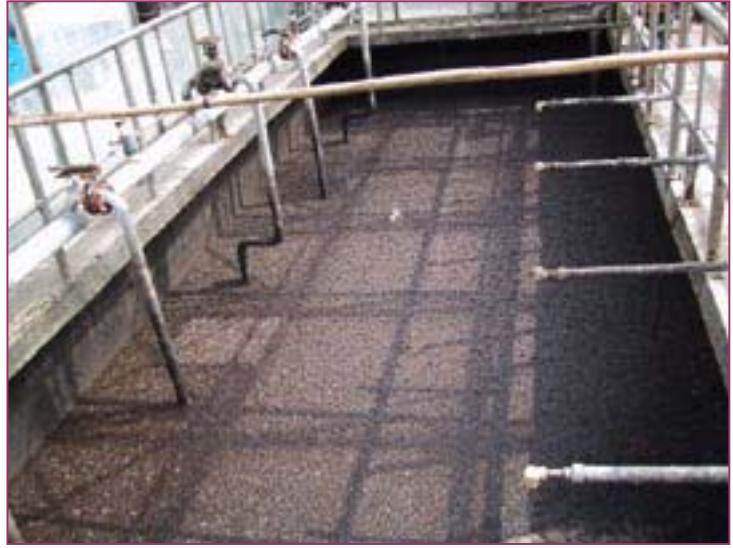
Primary Settling Basin
