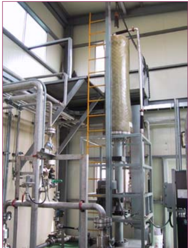
VSEP System installed for Hog Manure Treatment in Korea
