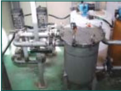
Bag Filter, Feed Pumps, & Chemical Metering Pumps for Cleaners
