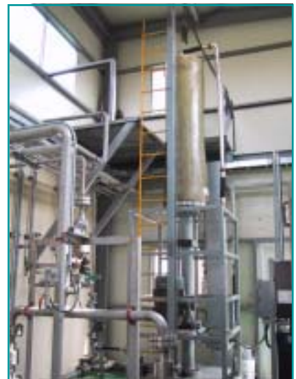
Kimhae Korea - V◇SEP New Logic's patented V◇SEP equipped with 1300 SF (120m 2 ) Reverse Osmosis membrane for the treatment of Hog Manure after a Sequencing Batch Bioreactor
